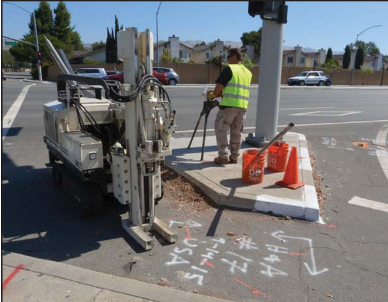
Photo 2. Refusal at Core 17 within the walkway portion of a current pedestrian island.
