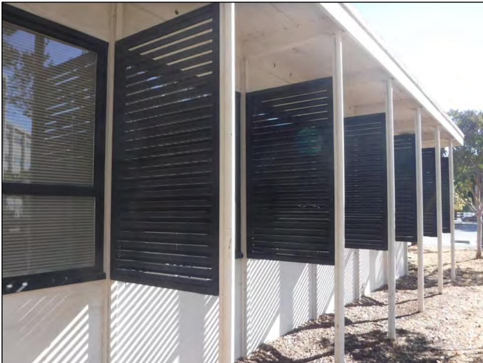
Photograph 3: Detail of windows and wood screens along façade, camera facing south, September 23, 2020.
