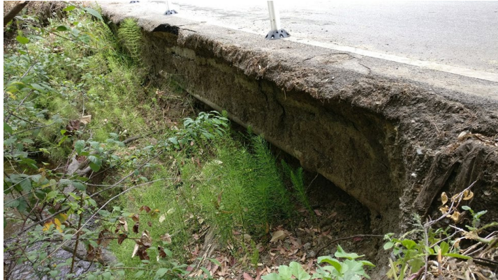
FIGURE 8. VIEW OF ARASTRADERO ROAD EMBANKMENT FOLLOWING 2016/2017 EROSION
