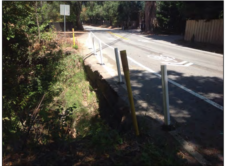
Photo 4. View of Arastradero Road facing northwest where scoured embankment occurs
