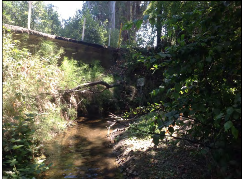
Photo 1. View of Los Trancos Creek where the channel flows below the scoured embankment
