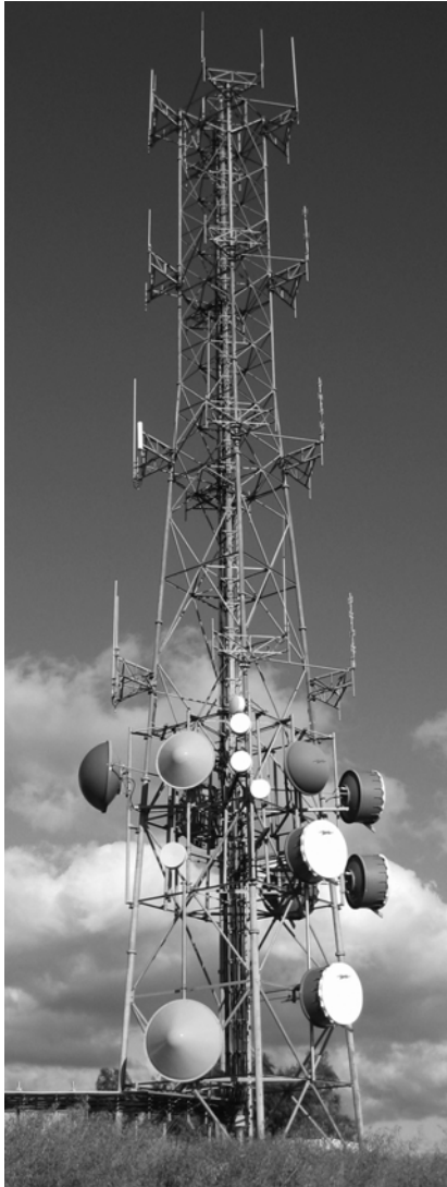
Above: One of several wireless radio communications towers located throughout the County in support of public safety and government operations.
