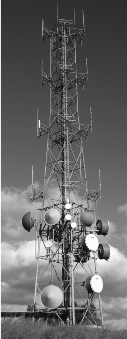
Above: One of several wireless radio communications towers located throughout the County in support of public safety and government operations.
