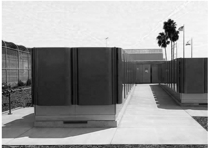
The Fuel Cell system installed at the Elmwood Correctional Facility is an 800 kilowatt system that generates 7 million kilowatt-hours of clean electricity each year, while saving the County an estimated $2.5 million over the 20 year Power Purchase Agreement under which it was installed.
