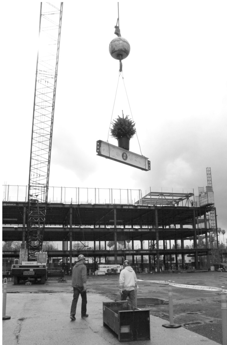
The tree is a traditional construction rite signifying that this beam is being placed at the highest point of the new Downtown Health Clinic.
