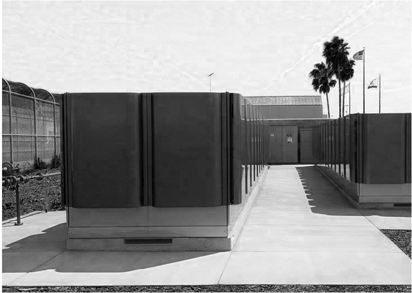
The Fuel Cell system installed at the Elmwood Correctional Facility is an 800 kilowatt system that generates 7 million kilowatt-hours of clean electricity each year, while saving the County an estimated $2.5 million over the 20 year Power Purchase Agreement under which it was installed.
